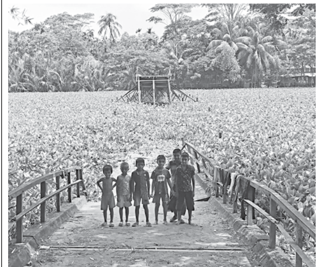
The bridge on Chawra canal, in Mohishdanga area of Barguna's Amtali upazila, collapsed on June 25.
