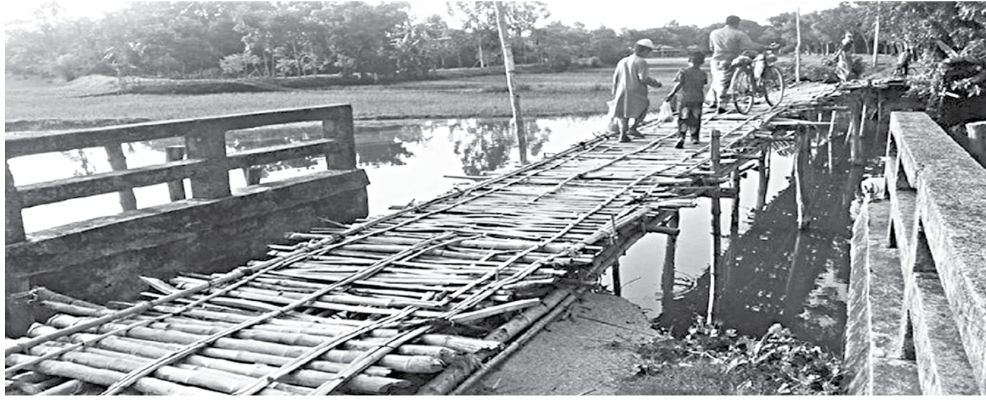
The makeshift bamboo footbridge that the villagers made after the approach road to the bridge, on Mohim canal in Nalchhapra village of Netrakona's Kalmakanda upazila, was washed away in flash floods about four years ago.
