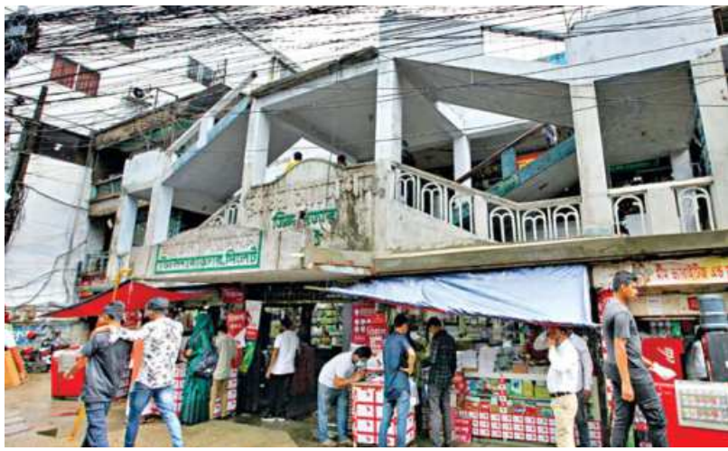
Although the owners want to demolish Raja Mansion, as the structure was deemed vulnerable to earthquakes, tenants are opposing the move. This photo was taken yesterday.
