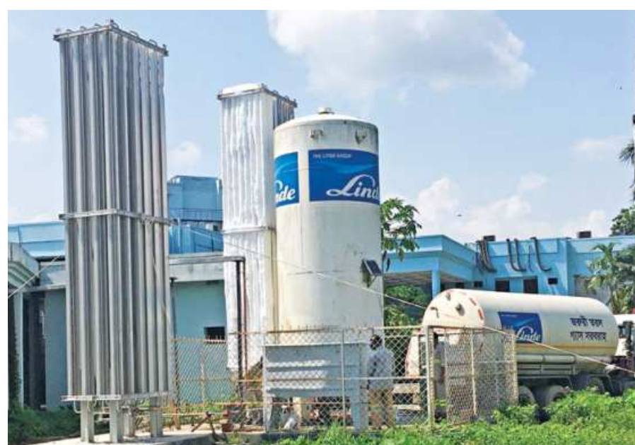
Rajshahi Medical College authorities have installed a new liquid oxygen vaporiser for uninterrupted supply and increasing oxygen pressure to Covid-19 patients. The vaporiser -- the hospital's second -- will help the authorities to extend wards for patients. This photo was taken yesterday.
