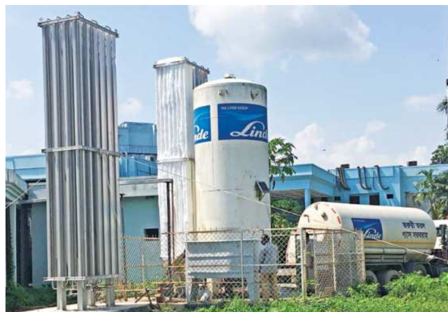
Rajshahi Medical College authorities have installed a new liquid oxygen vaporiser for uninterrupted supply and increasing oxygen pressure to Covid-19 patients. The vaporiser -- the hospital's second -- will help the authorities to extend wards for patients. This photo was taken yesterday.
