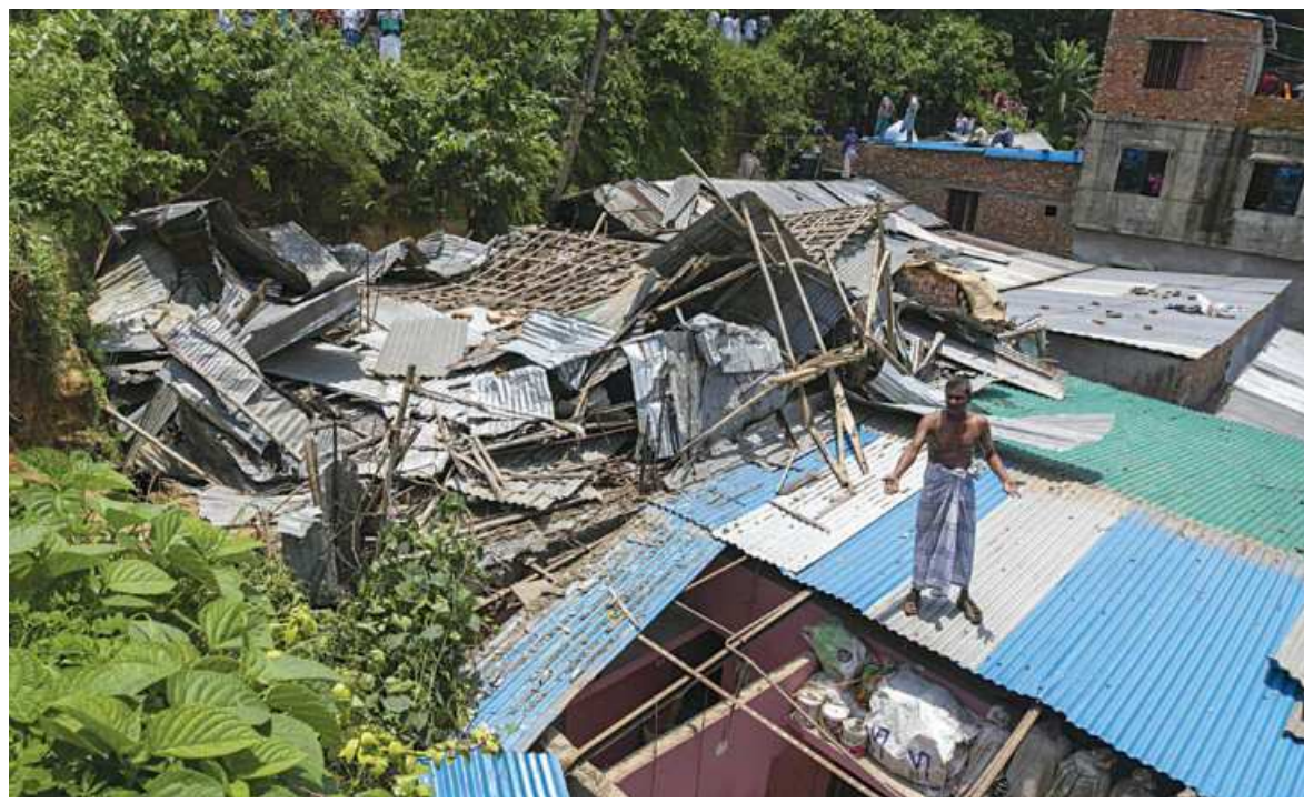
A man stands on the roof of his torn down house after Chattogram district administration evicted people living on the hill slopes ignoring risks of landslides. The photo was taken in Lal Khan Bazar of the port city.
