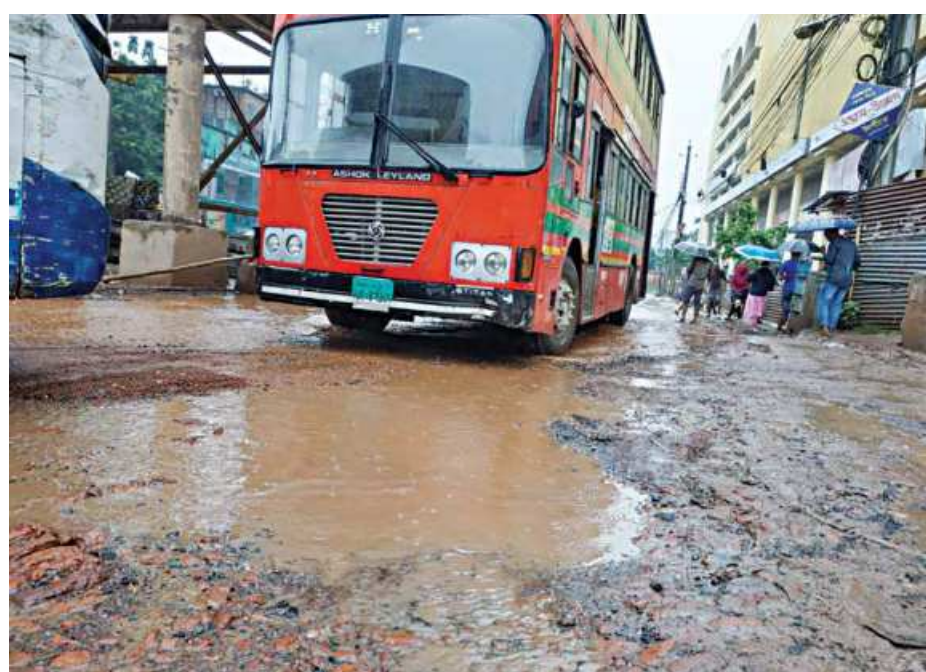
Vehicles have to go slow on the portion of road between Dhaka's Abdullahpur to Chandana Chowrasta of Gazipur on the Dhaka-Mymensingh highway as rain water stagnates in potholes. The slow traffic also causes traffic jams. The photo was taken from Tongi Station Road area yesterday.
