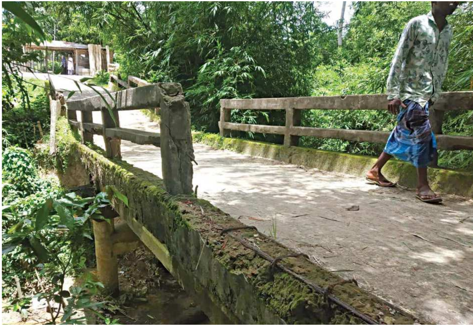
A broken bridge on the local road in Alisarkul area of Moulvibazar's Srimangal upazila poses fatal accident of commuters.
