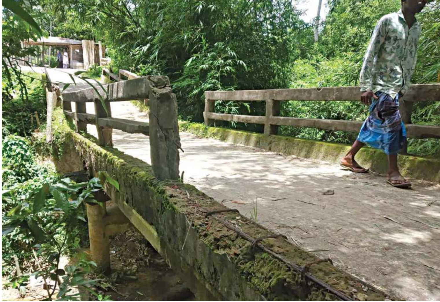
A broken bridge on the local road in Alisarkul area of Moulvibazar's Srimangal upazila poses fatal accident of commuters.
