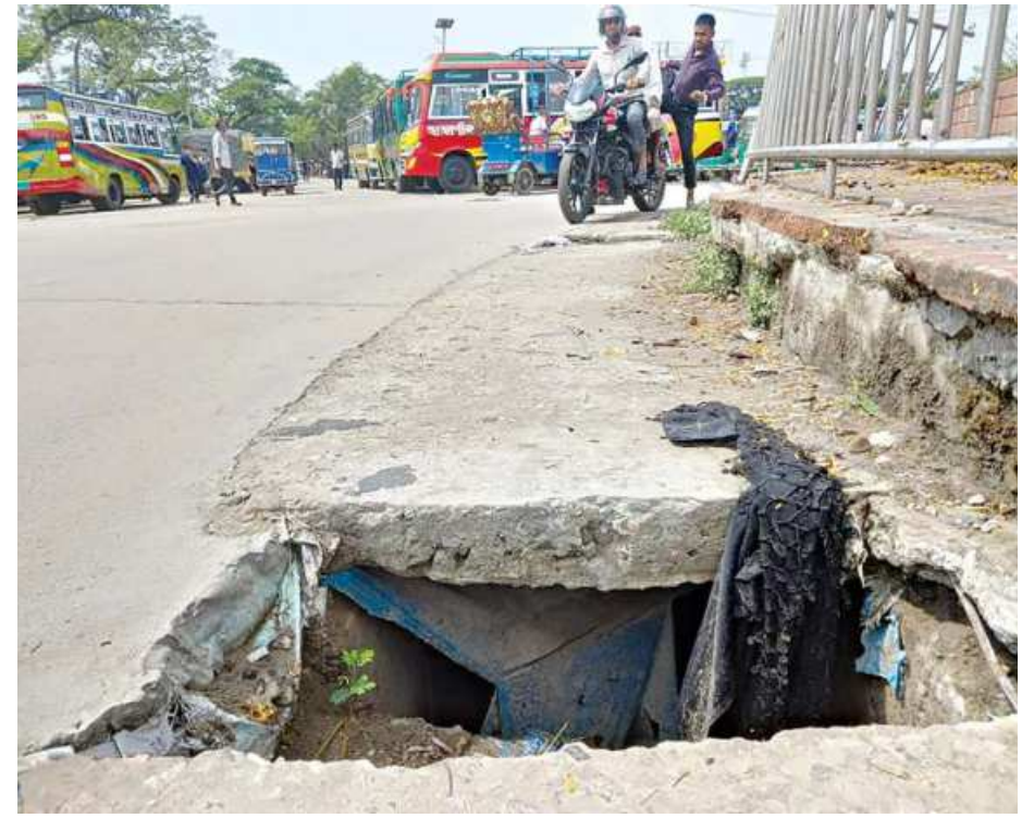
A section of the damaged concrete slabs around the Muktijoddha Chatter on Sylhet-Dhaka highway in Sherpur Bazar of Moulvibazar Sadar upazila.
