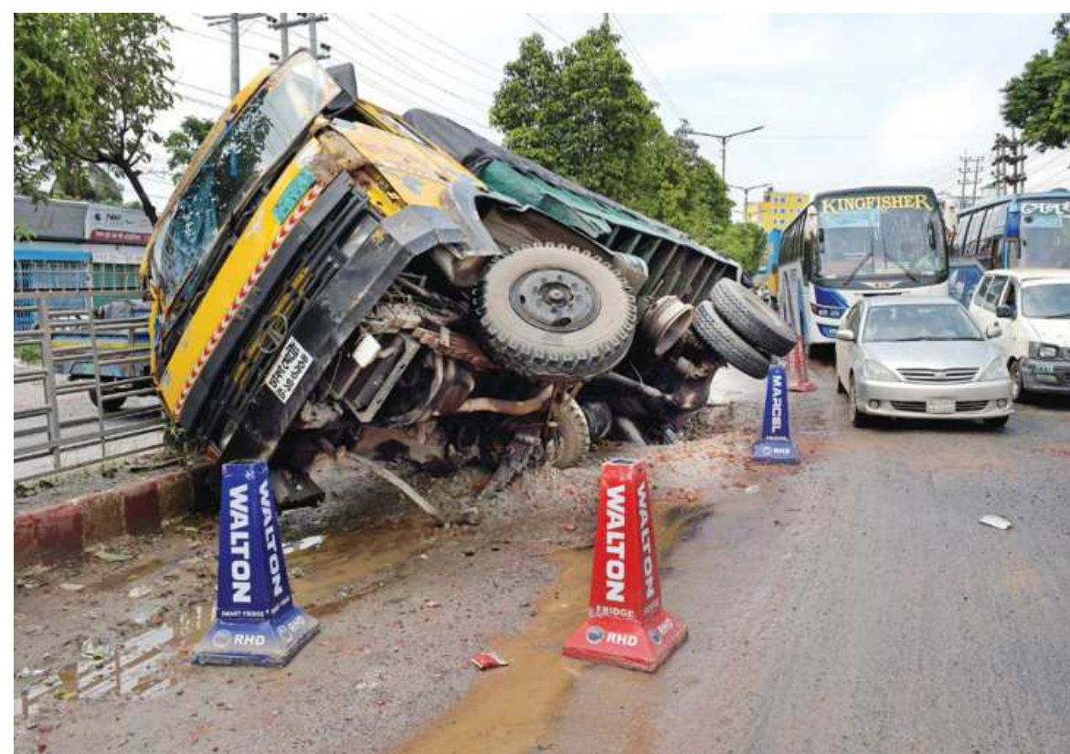
This pickup van turned sideways on the Dhaka-Aricha highway near Savar Bazar bus stand on Thursday night. Locals said the accident occurred due to there being no safety barriers around a road development works spot. Fortunately, no casualties have been reported, though risks persisted as of yesterday morning as the vehicle was left lying without any protection, leaving it prone to tumbling over.
