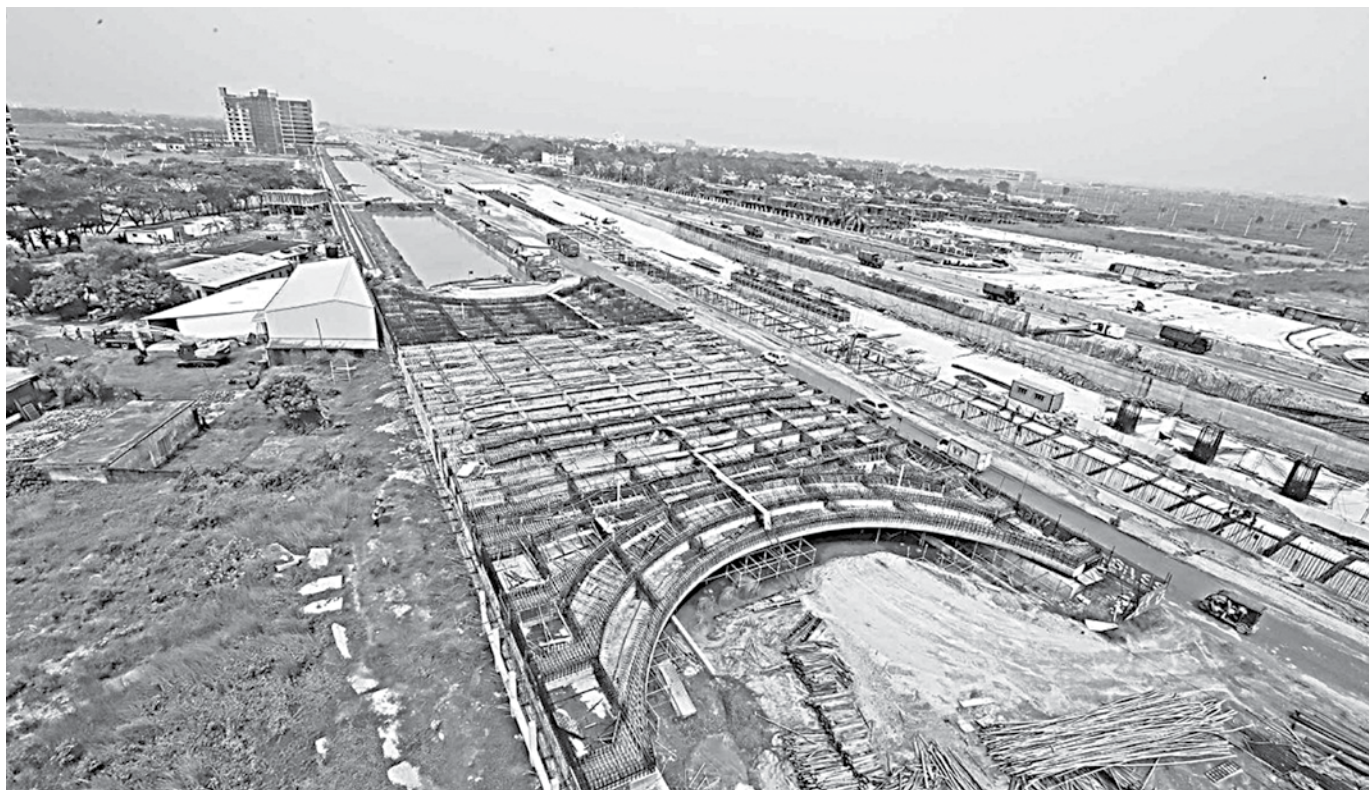
A massive development work at the 300-foot Purbachal Road is underway. The government is constructing an eight-lane expressway to connect Kuril with Kanchan Bridge via Purbachal. Besides, 100-foot canals are being built on both sides of the road from Kuril to the Balu River.
