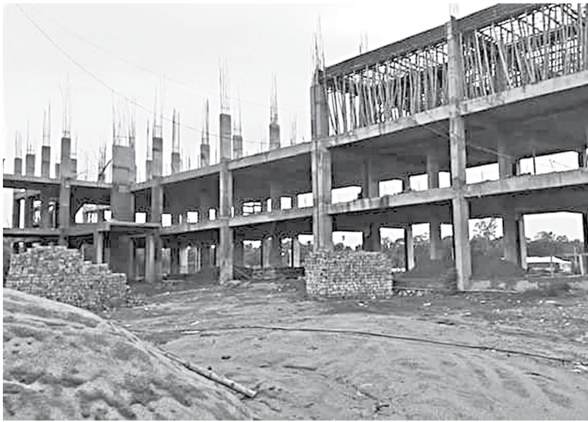
One of the two under-construction buildings of Taimush Ali Technical School and College in Bhabanipur area of Juri upazila in Moulvibazar. The contractor has been found to be using below par rod in the construction of both buildings of the institution.
