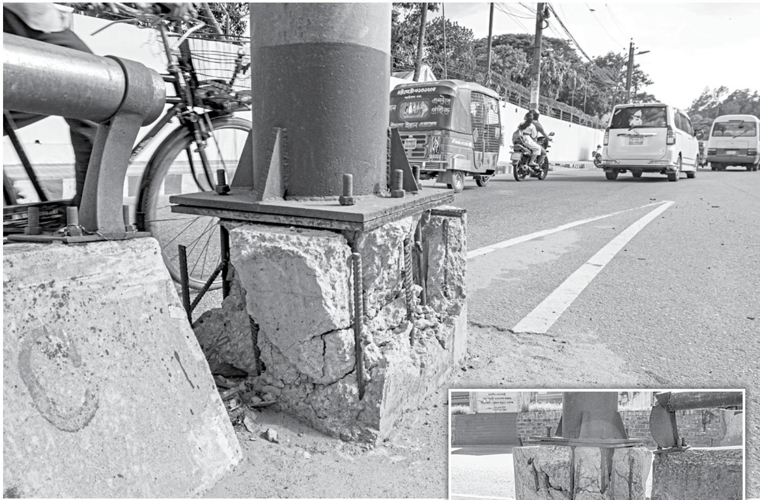
This pillar at the base of Chattogram city's Akhtaruzaman flyover might fall over any day, as the foundation is crumbling away. If something is not done, this could lead to a major accident, as vehicles drive past the structure non-stop. The photos were taken recently from Lalkhan Bazar area.
