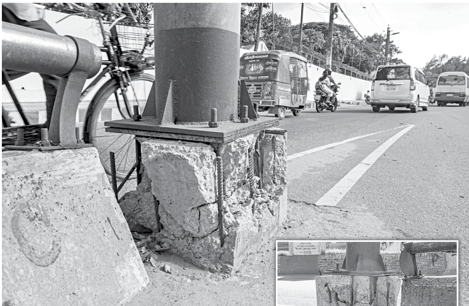
This pillar at the base of Chattogram city's Akhtaruzaman flyover might fall over any day, as the foundation is crumbling away. If something is not done, this could lead to a major accident, as vehicles drive past the structure non-stop. The photos were taken recently from Lalkhan Bazar area.
