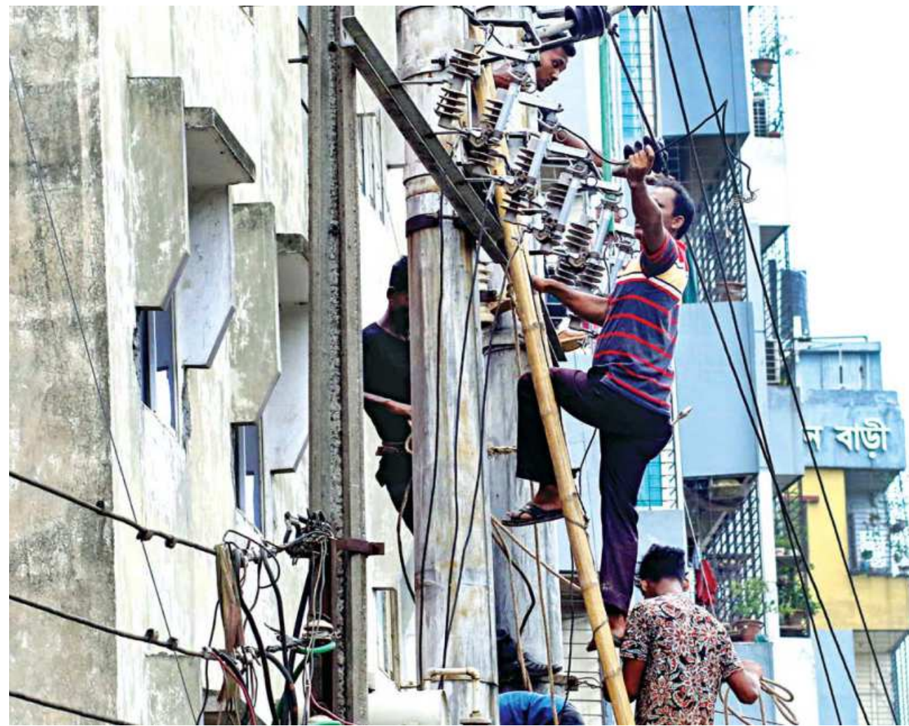
Without a harness or any other safety measures, two electricians are working on a very high volt transformer in the capital's Farm Gate area. A momentary lapse in concentration or loss of footing can lead to tragedies in such situations.
