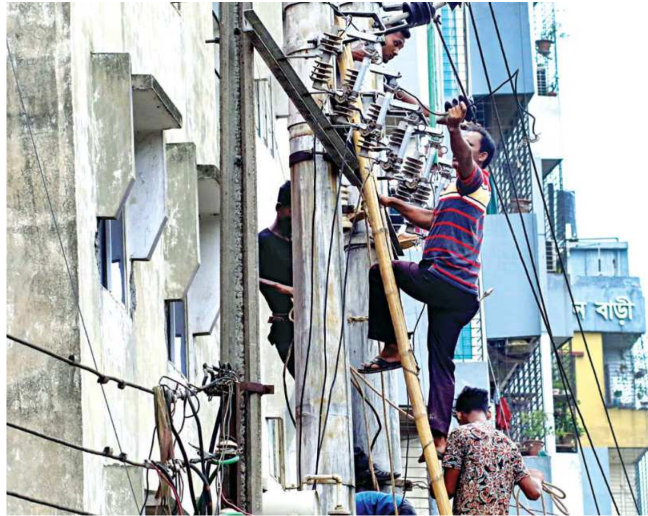
Without a harness or any other safety measures, two electricians are working on a very high volt transformer in the capital's Farm Gate area. A momentary lapse in concentration or loss of footing can lead to tragedies in such situations.
