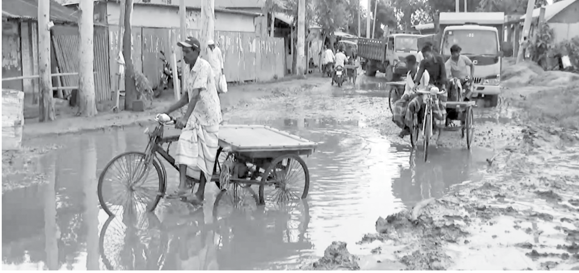
The damaged stretch on Madhupur road from Sagardighi in Tangail's Ghatail upazila.
