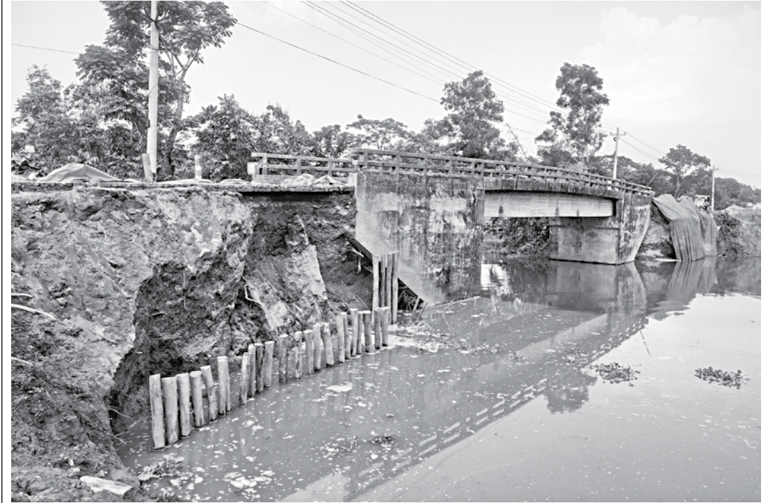
Roads and Highways Department in Kishoreganj recently placed wood logs to stop further erosion of an approach road to this bridge on Bogaputa canal in Ishwarganj upazila of Mymensingh. PHOTO: COLLECTED
