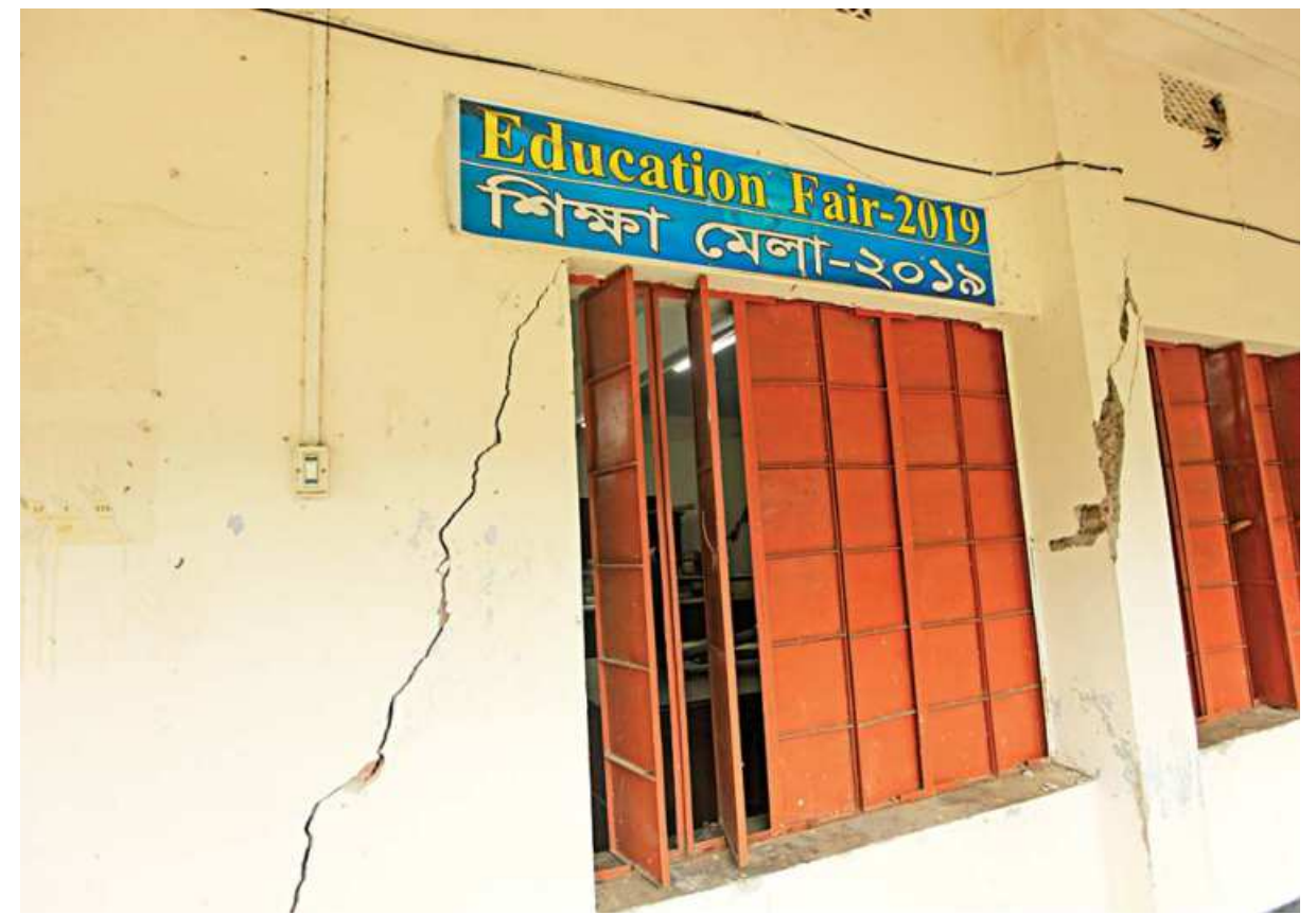
Cracks developed on a two-storey academic building of the century-old Raja Girish Chandra High School after a mild tremor of magnitude 3.8 jolted Sylhet city on Monday evening. After inspecting the building yesterday, authorities declared it risky and are planning to demolish it.
