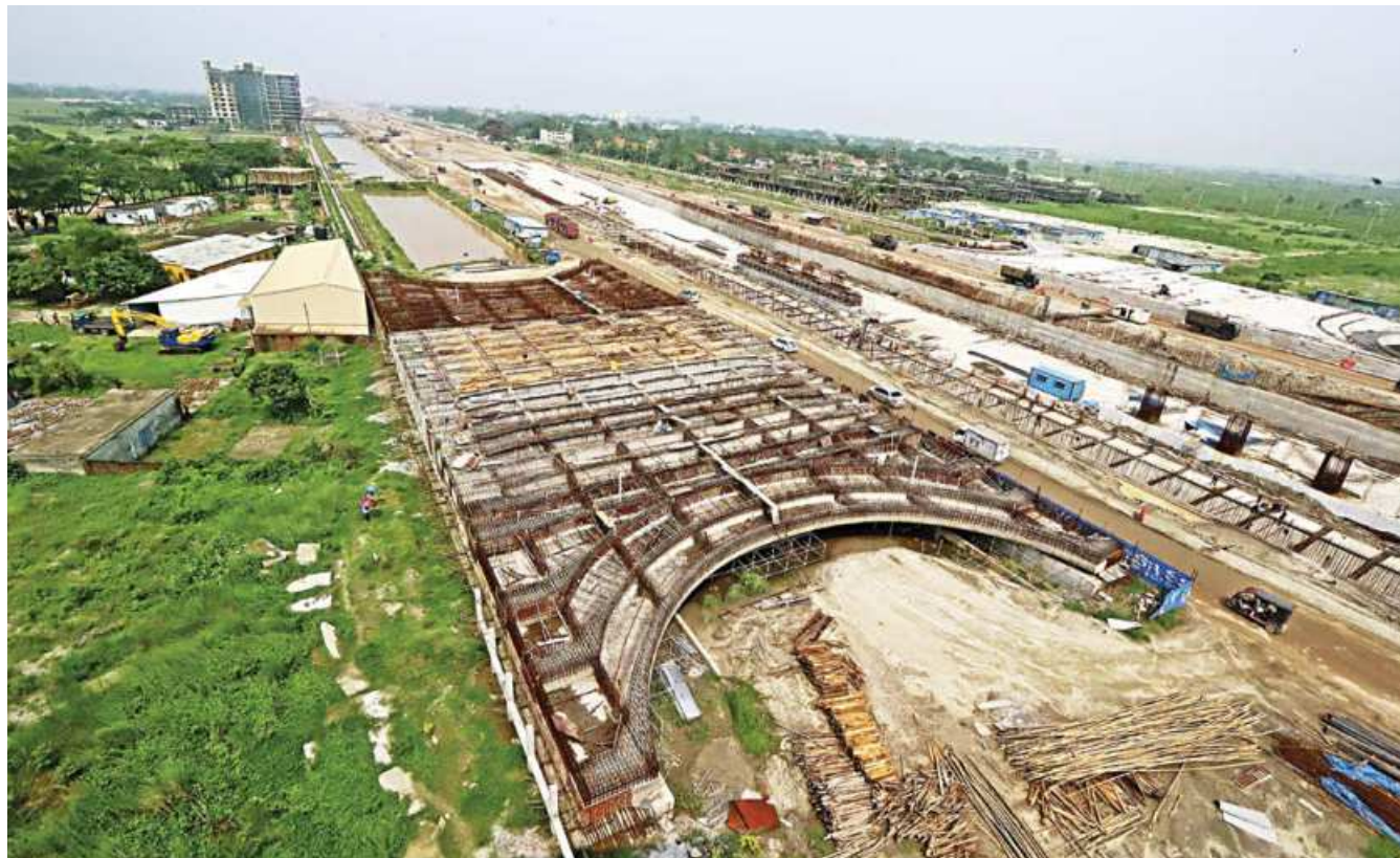
A massive development work at 300-foot Purbachal Road is underway. The government is constructing an eight-lane expressway to connect Kuril with Kanchan Bridge via Purbachal. Besides, 100-foot canals are being built on both sides of the road from Kuril to the Balu river. The photo was taken on Monday.
