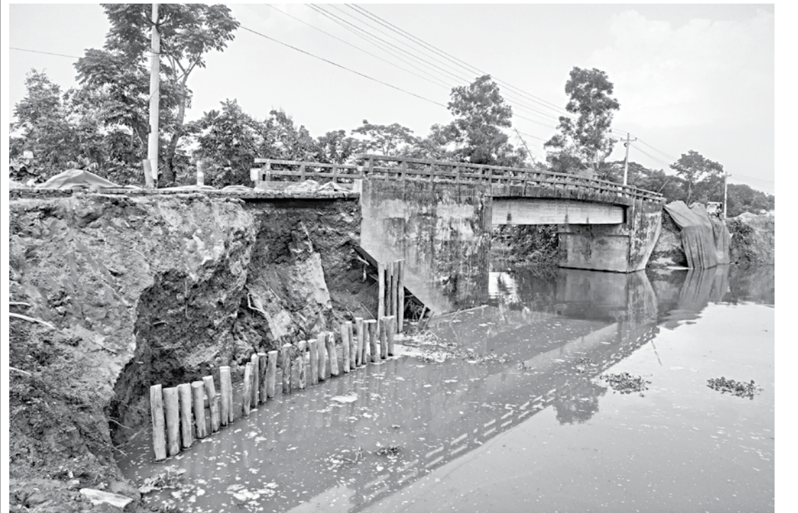
Roads and Highways Department in Kishoreganj recently placed wood logs to stop further erosion of an approach road to this bridge on Bogaputa canal in Ishwarganj upazila of Mymensingh.
