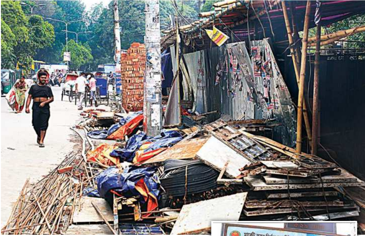
It must be great news for residents of the capital's Azimpur that Dhaka South City Corporation is constructing a 'modern' market in their neighborhood. But if those elected to ensure public interest violate it, as is evident by the strewn-about construction material on the footpath and road, then who does one complain to? DSCC ward-26 councillor is supervising the project, as announced on a board on the site, inset. The photos were taken yesterday.
