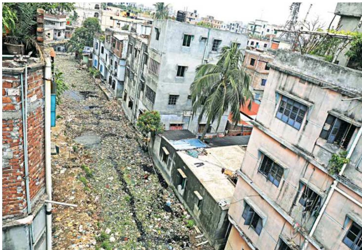
People discard bottles, containers, and polythene bags into the capital's Shyampur canal, polluting the water and clogging the canal. Water stagnates and the canal becomes a breeding ground for mosquitos. Its cleanup and development work has been halted for a long time. The photo was taken on Saturday. PHOTO: AMRAN HOSSAIN
