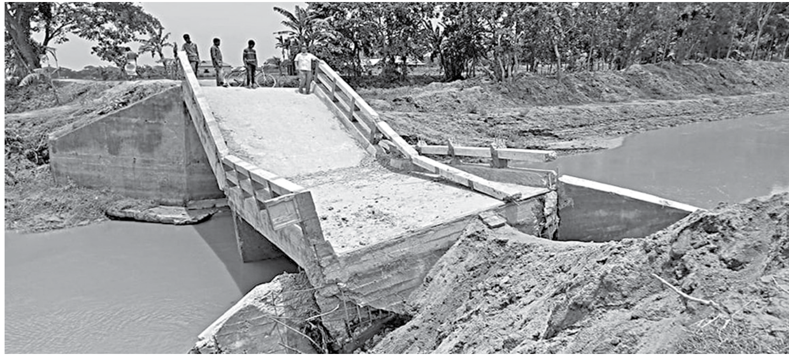
The Borakhali Bridge that collapsed on May 26. It was built over Borakhali canal in 2017-2018 fiscal year.
