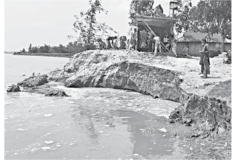
Roads, educational institutions, religious institutions, dwellings and cultivable lands are being devoured by the Teesta River at Bajra Union of Ulipur upazila in Kurigram.
