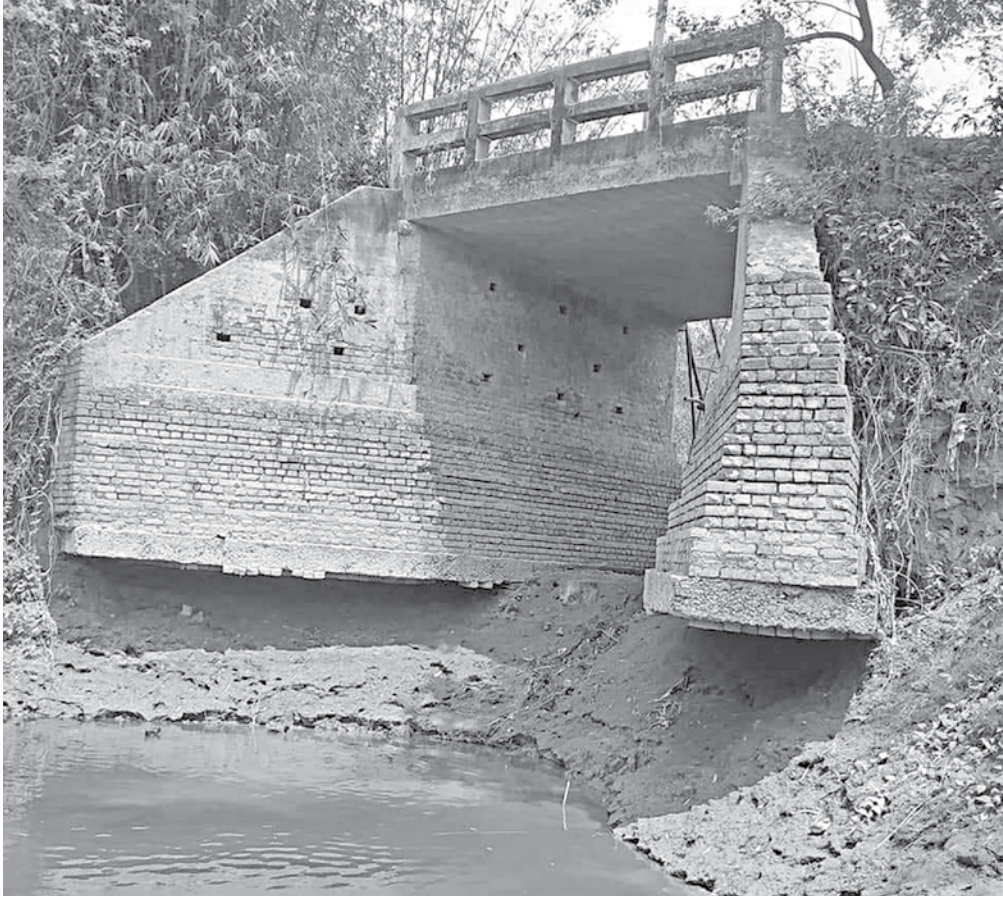
An old bridge at Hilora Adabari village under Mohera union in Tangail's Mirzapur upazila has remained in a vulnerable condition posing threat to a fatal accident.
