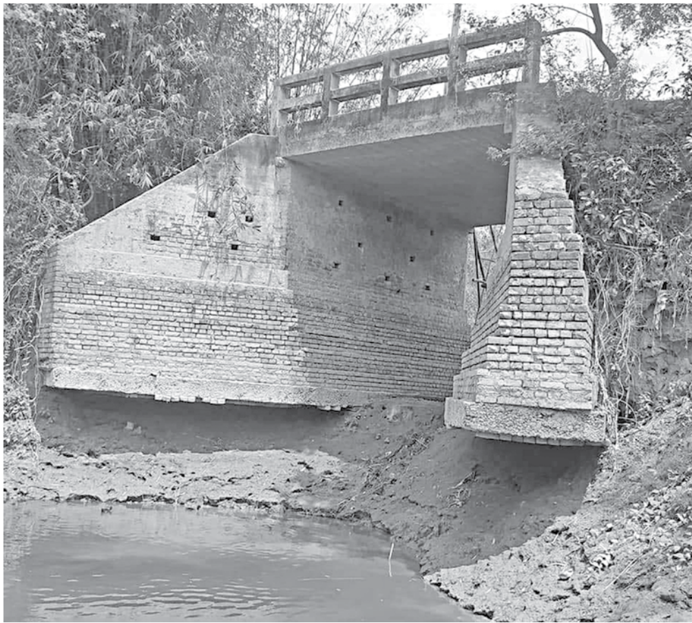
An old bridge at Hilora Adabari village under Mohera union in Tangail's Mirzapur upazila has remained in a vulnerable condition posing threat to a fatal accident.
