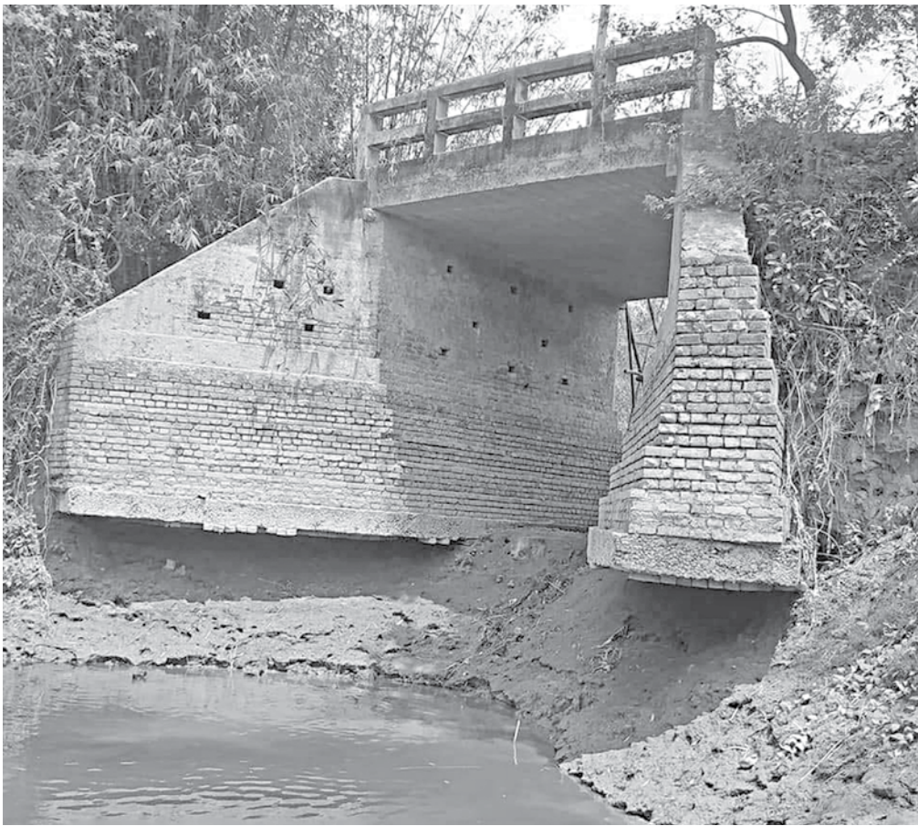
An old bridge at Hilora Adabari village under Mohera union in Tangail's Mirzapur upazila has remained in a vulnerable condition posing threat to a fatal accident. PHOTO: STAR
