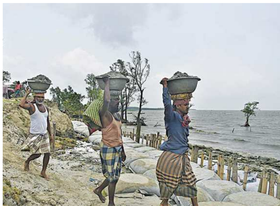
Villagers in Barguna's Patharghata upazila carrying baskets filled with sand to be put in geo bags in order to repair an embankment along the Baleswar river that was breached by tidal surges during Cyclone Yaas. The photo was taken on Monday.
