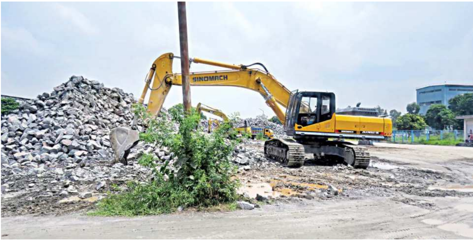
A hydraulic crane is being used for loading rocks on the site of Maddhapara Granite Mining Company Ltd in Dinajpur.
