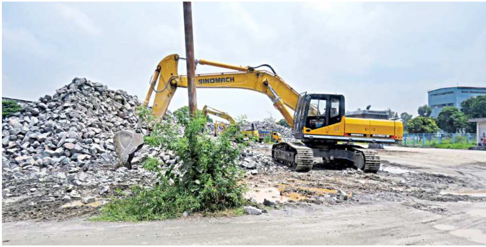
A hydraulic crane is being used for loading rocks on the site of Maddhapara Granite Mining Company Ltd in Dinajpur.
