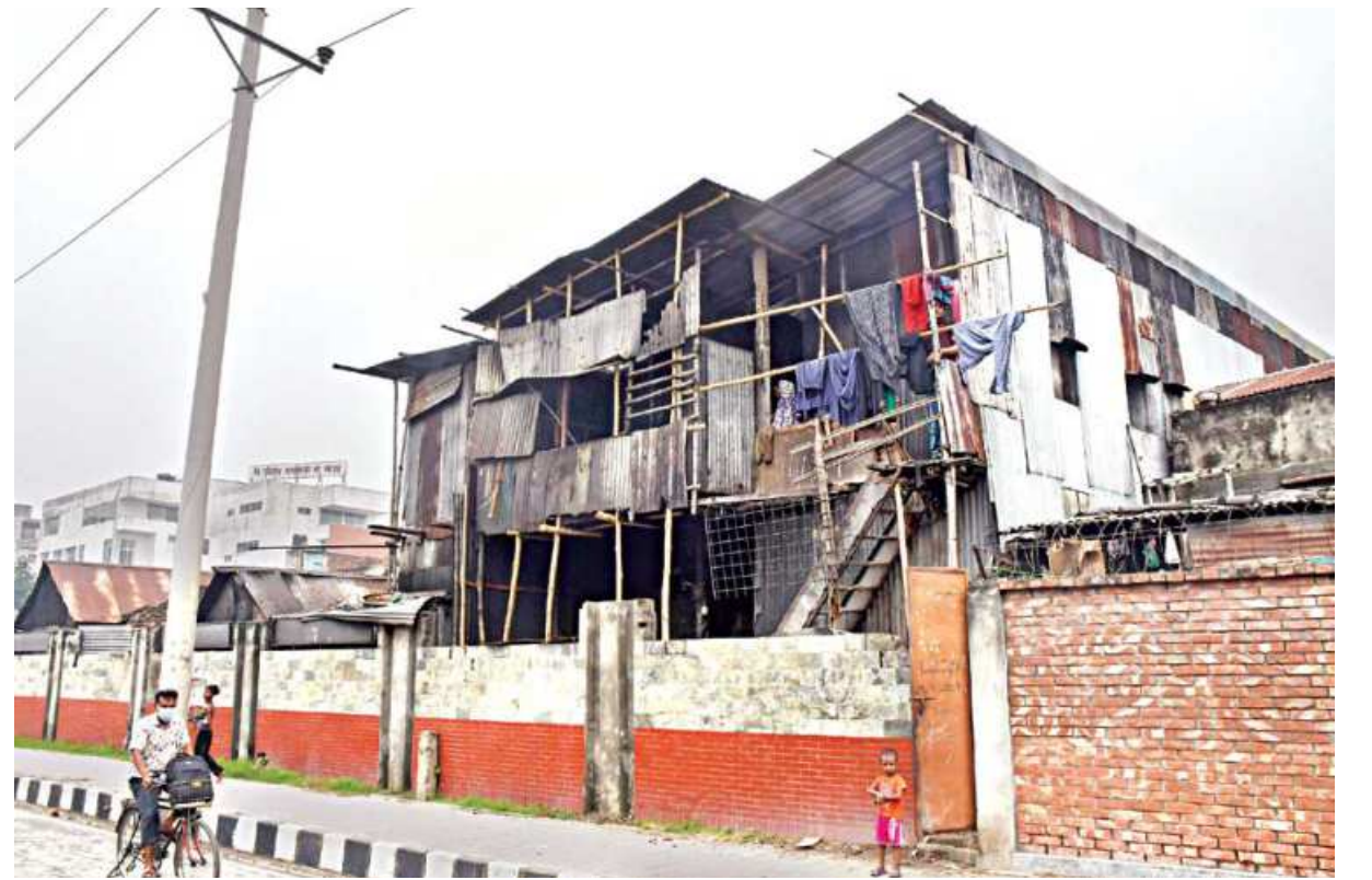
This "two-storied" house stands on poles and a platform made out of bamboo, and its walls and roof are made of corrugated tin sheets that appear to be rusty and repurposed. A blatant violation of any housing safety guideline, this fragile, risky structure stands not on the outskirts of the capital but in the rather central Moghbazar area. The photo was taken yesterday.
