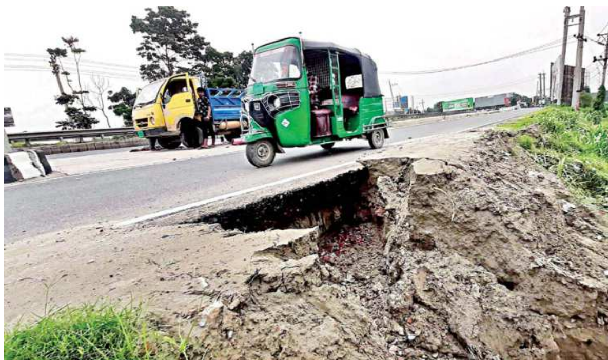
A big chunk of earth along Dhaka-Tangail highway was eroded by rain water yesterday, making this part of the road risky. The photo was taken in Ashekpur Bypass area of Tangail.
