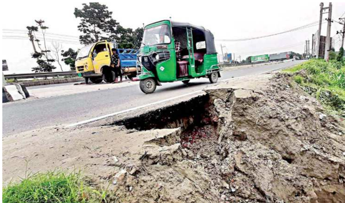
A big chunk of earth along Dhaka-Tangail highway was eroded by rain water yesterday, making this part of the road risky. The photo was taken in Ashekpur Bypass area of Tangail.
