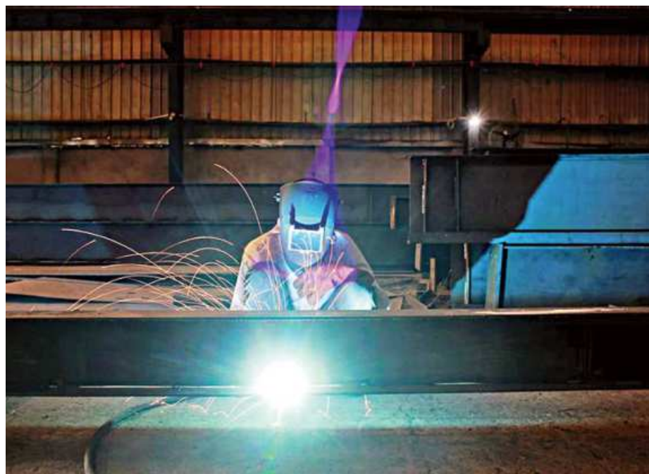
A labourer welds an iron pillar at a building material factory in an industrial area in Dasna, in the central Indian state of Uttar Pradesh.
