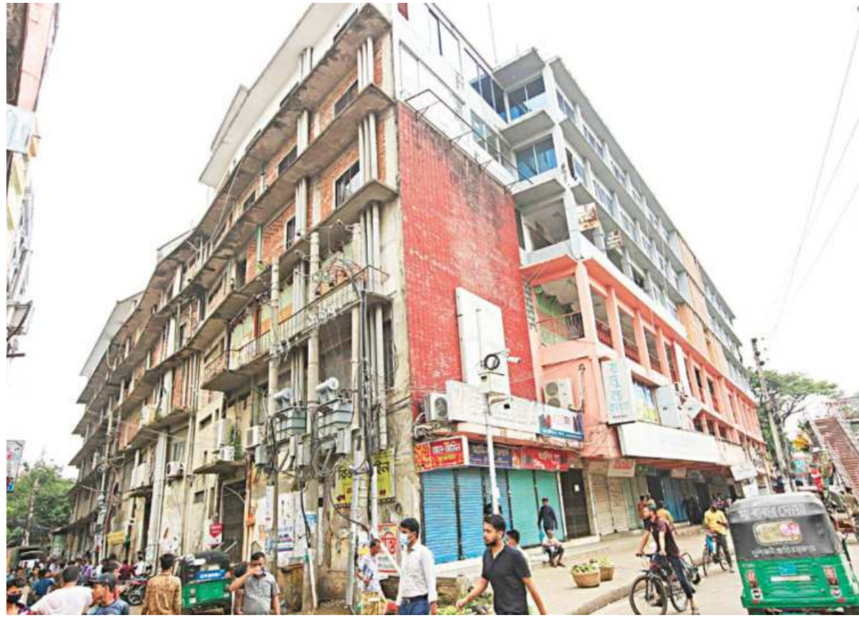
Following consecutive days of earthquakes, Sylhet City Corporation has decided to close down six risk-prone markets, including this Modhubon Market in Bandar Bazar for 10 days, starting from yesterday till June 9. After receiving the mayor's orders, members of the market committees sat for a meeting yesterday.
