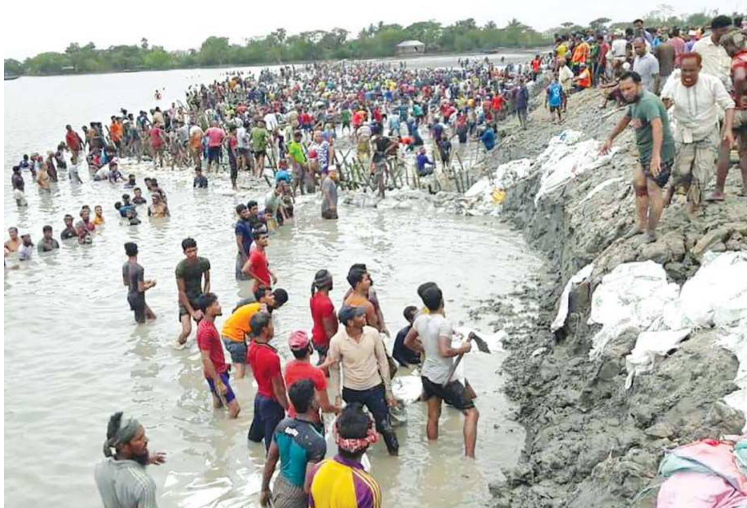
Locals voluntarily repair an embankment in Dashaia area of Khulna's Koyra upazila yesterday. The dam was damaged due to tidal surges caused by cyclone Yaas. At least 38 villages have been flooded as water from a river entered in the localities.
