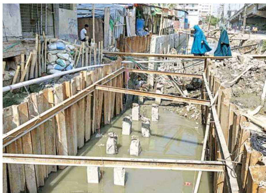
People living in Muradpur intersection area of Chattogram city have to cross this dangerous trench by walking on planks. A lengthy work on the drainage there has forced the people of the neighbourhood take the risk every day. The photo was taken yesterday.
