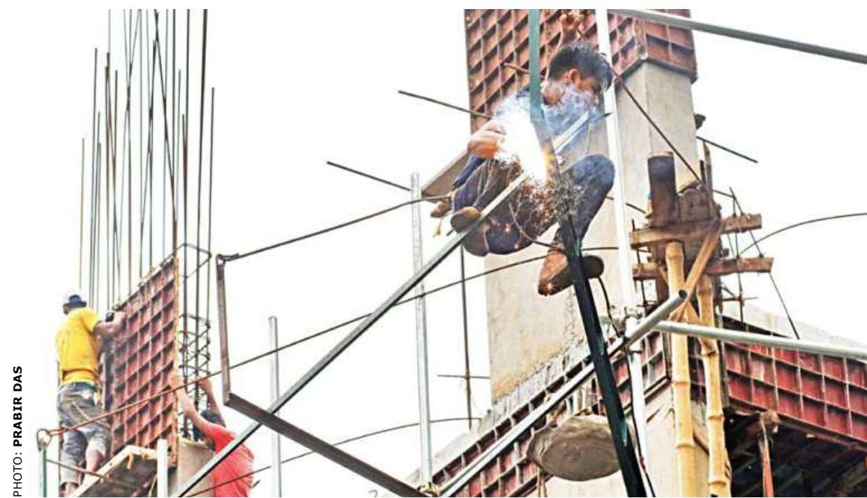
A worker barely balances himself on two thin rods, welding a safety shed on the fifth level of an under-construction building to prevent any debris from falling on passers-by. But there is no safety equipment, or even a helmet for the worker himself as he risks his life at the site. This photo was taken from Kazi Nazrul Islam Avenue in Dhaka recently.
