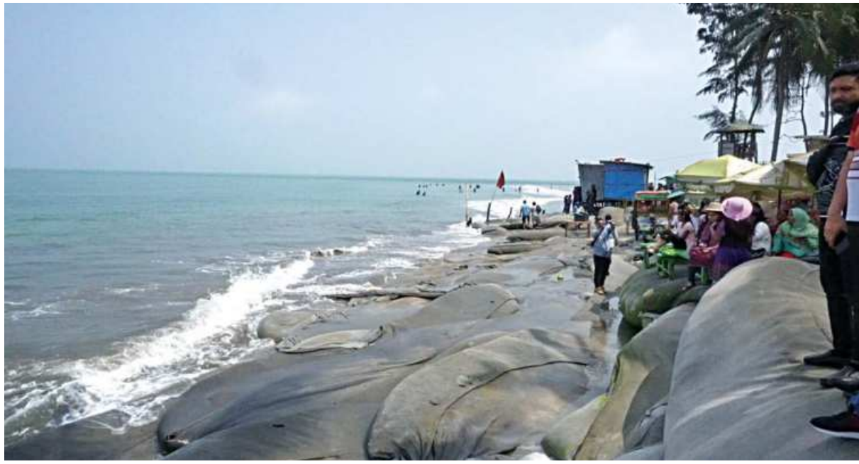
The northern beach of St Martin's Island where geotextile bags filled with sand from the same location is causing further erosion of the beach. The Department of Environment said they filed a case against the local union parishad chairman for placing the bags without obtaining necessary authorisation.
