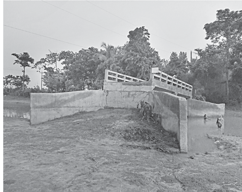
The Tk 28-lakh bridge lying useless without any road for over five years, near Uttarhati village in Ajmeriganj upazila of Habiganj.
