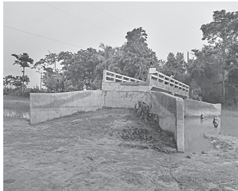
The Tk 28-lakh bridge lying useless without any road for over five years, near Uttarhati village in Ajmeriganj upazila of Habiganj.
