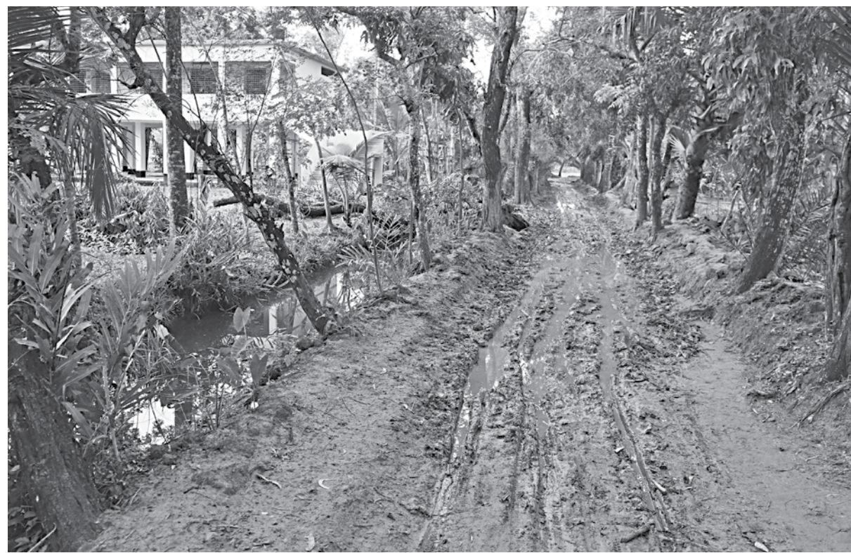
After the LGED contractor removed the upper layer of soil from the road -- in Pirojpur's Indurkani upazila -- and abandoned work six months ago, stagnant water from recent spells of rain has turned it into a long trench filled with mud.
