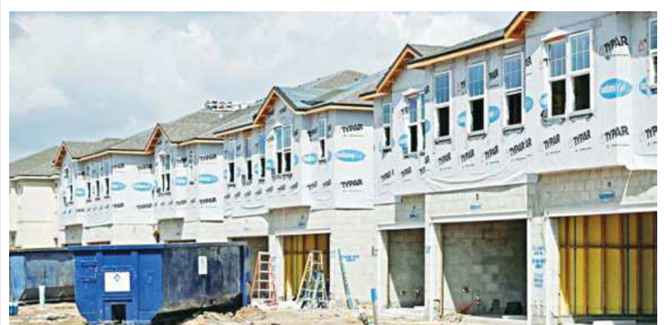
New townhomes are seen under construction while building material supplies are in high demand in Tampa, Florida.
