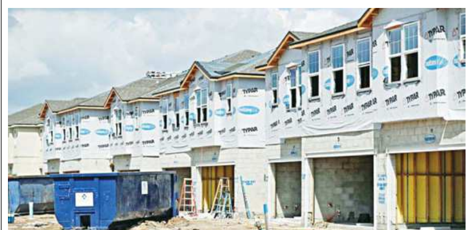
New townhomes are seen under construction while building material supplies are in high demand in Tampa, Florida.
