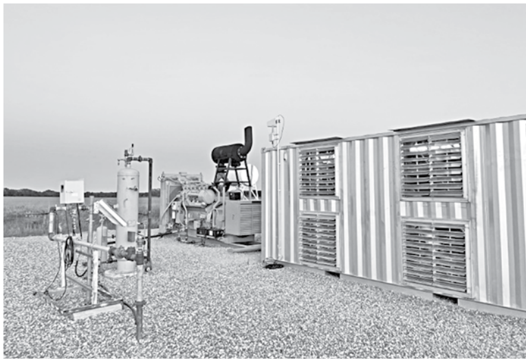
A handout photo from Giga Energy Solutions shows a natural gas generator powering a bitcoin mining centre in north Texas in May.
