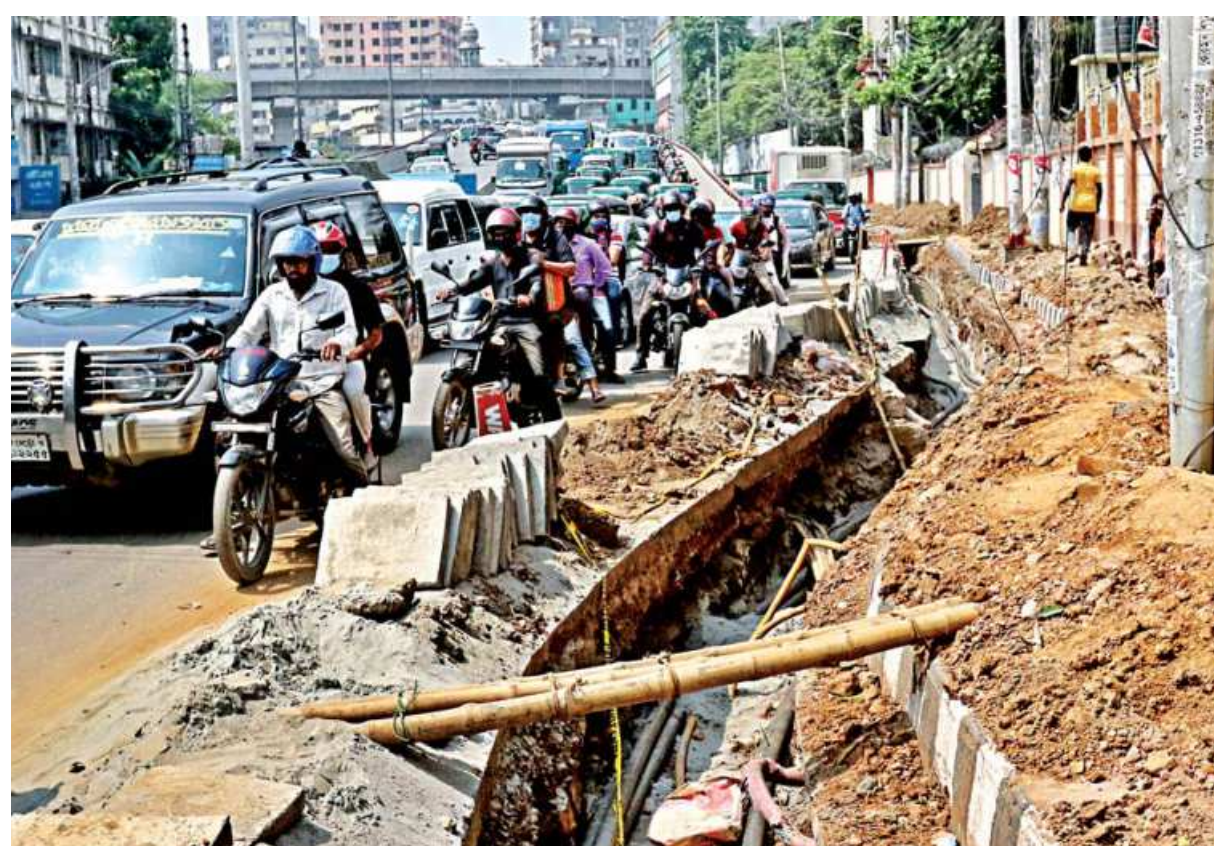
A significant portion of the Moghbazar-Kakrail road is being dug for development works. Though this was less of a problem during the "strict" lockdown, now that movement guidelines are relaxed, commuters of the street are suffering massively due to the obstruction.
