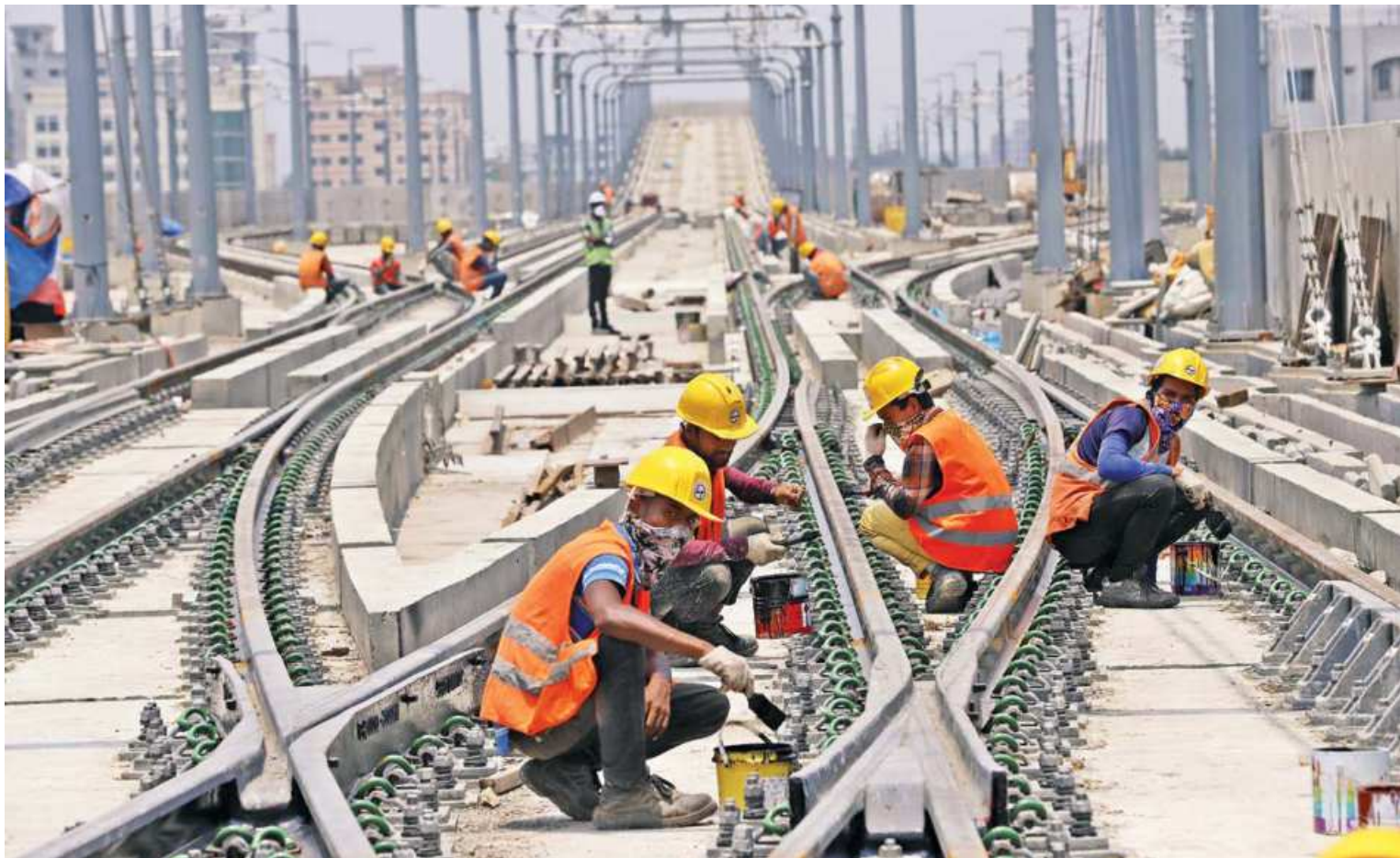
Workers putting the finishing touches on the tracks at the Uttara North metro rail station in the capital. Officials are planning to conduct a test run of the country's first metro rail service -- the Mass Rapid Transit-6 -- which will stretch from this station in the capital's north to Motijheel in the south. The photo was taken on Saturday.
