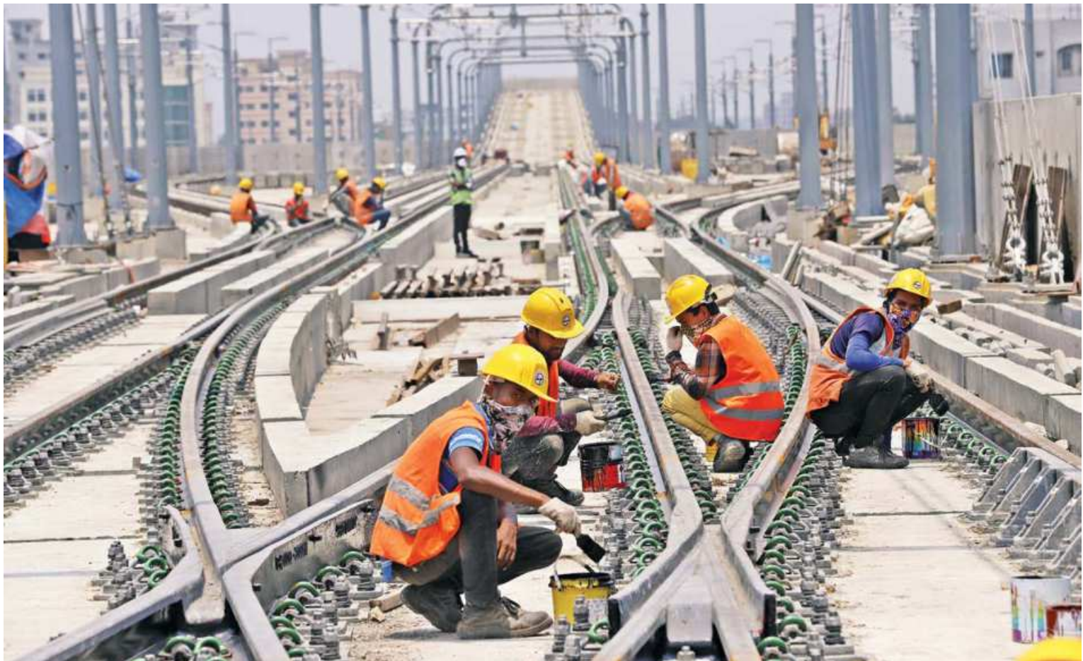
Workers putting the finishing touches on the tracks at the Uttara North metro rail station in the capital. Officials are planning to conduct a test of the country's first metro rail service -- the Mass Rapid Transit-6 -- which will stretch from this station in the capital's north to Motijheel in the south. The photo was taken on Saturday.
