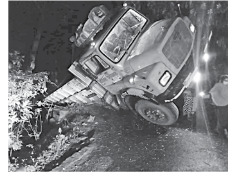
The worn-out bridge on a canal in Tangail's Nagarpur upazila collapses when a sand-laden truck was crossing it on Friday night.
