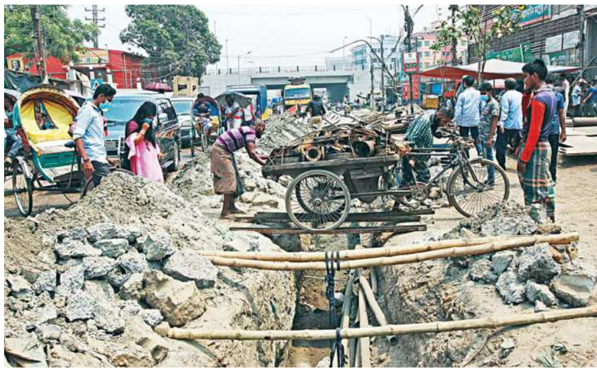
Two men moving a loaded rickshaw van across a trench using precariously placed planks near Postogola fire station in the capital yesterday. Residents and businesses said the trench, dug for the maintenance of utility pipes about seven months ago, has made it difficult for them to use the road.
