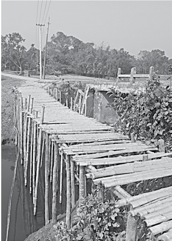
This bridge over the Buribhairab river on Chowgachha-Barobazar road in Jhenidah's Kaliganj upazila is lying unrepaired for long.
